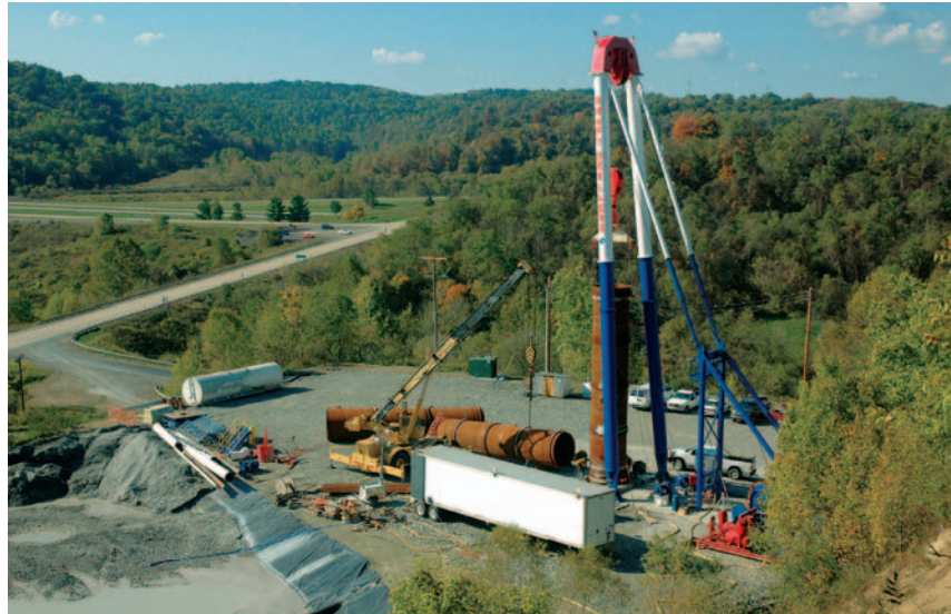
Shaft drilling operations are conducted from the surface with only a few miners.
